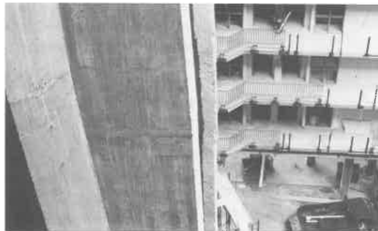
SHODDY CONSTRUCTION at Charleston's Embassy Suites included these out-of-line nine-story concrete elevator shafts.
