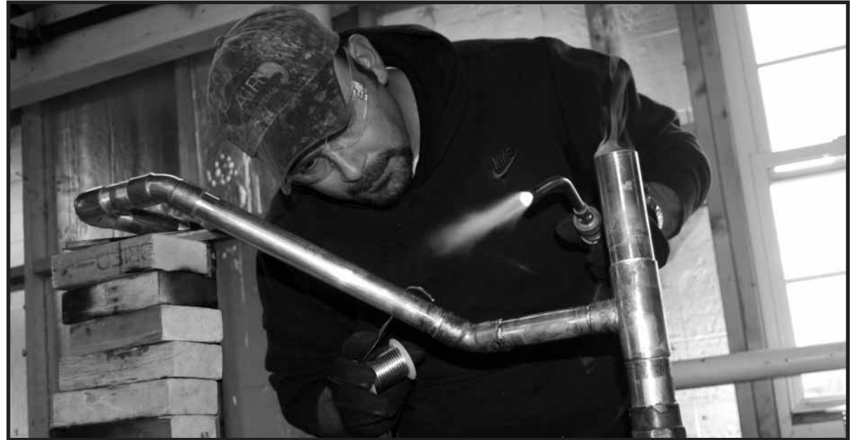
GEORGE LAWSON FROM Local 625 Charleston is soldering refrigeration piping as part of the HVAC contest.
