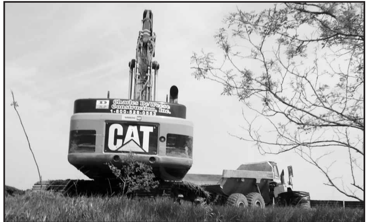
KENTUCKY CONTRACTOR Charles DeWeese Construction Inc., works on the site of the Macy's distribution center project funded by a forgivable state loan of $5 million to Macy's.
