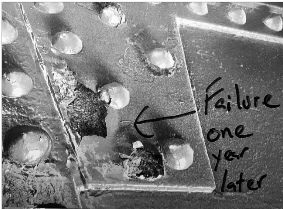
This picture of rust came from recent pictures taken by Painter Representative Dave Bland at the Yeager Bridge in Kanawha County. The WV Turnpike Authority paid almost $1 million to have the bridge repainted less than one year ago.
